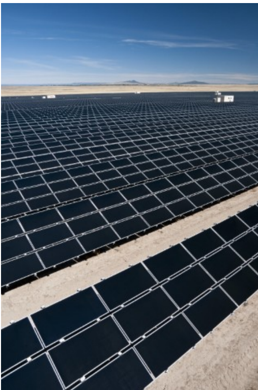
Below, a well-maintained utility-scale solar plant produces energy (and revenue) for its design life.
