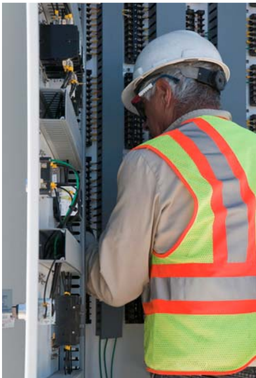
Above, an O&M provider monitors plant systems for prompt reactions to output issues.
